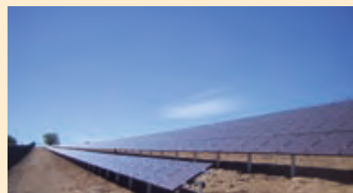
PV plant Lameelas, Portugal
