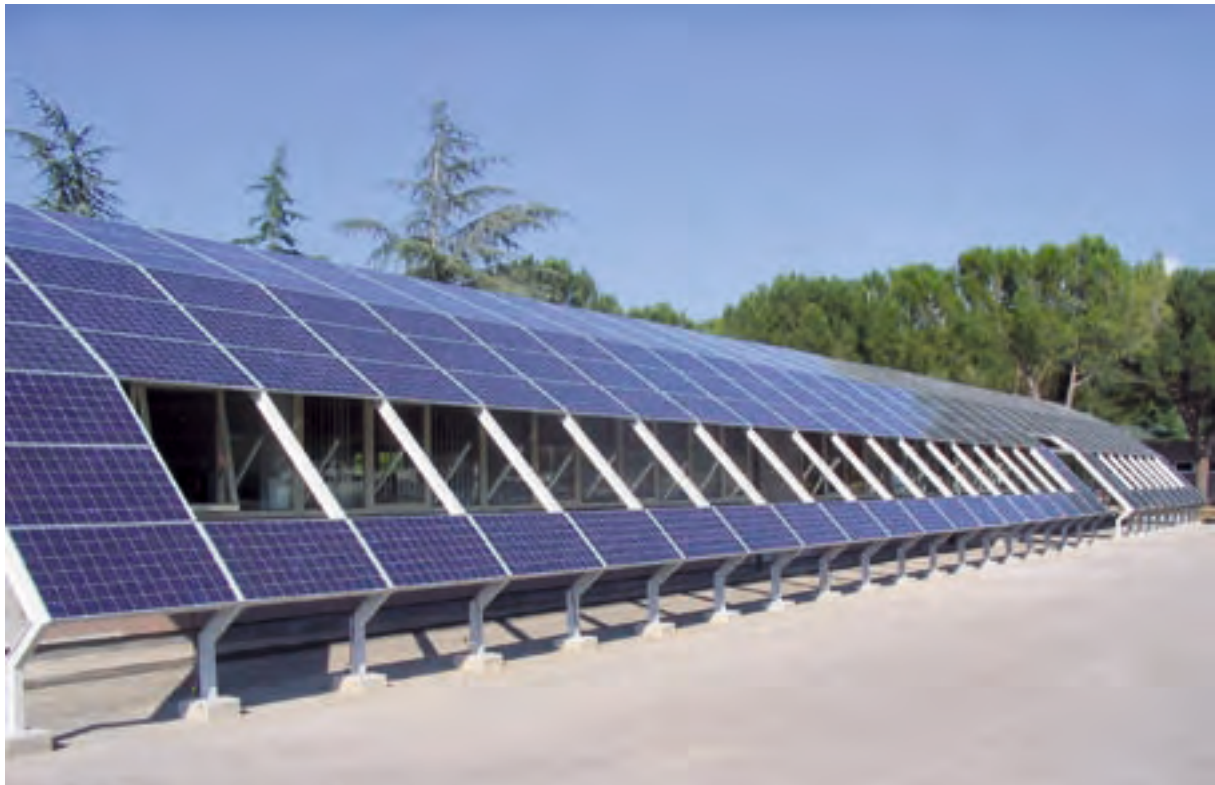
40 kW PV plant, Narni, Italia (courtesy of GSE)
