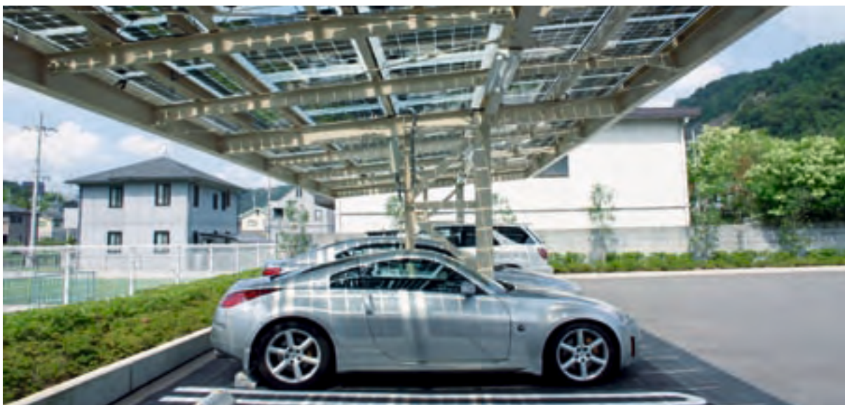
PV system at parking lot in Fujipream, Japan
