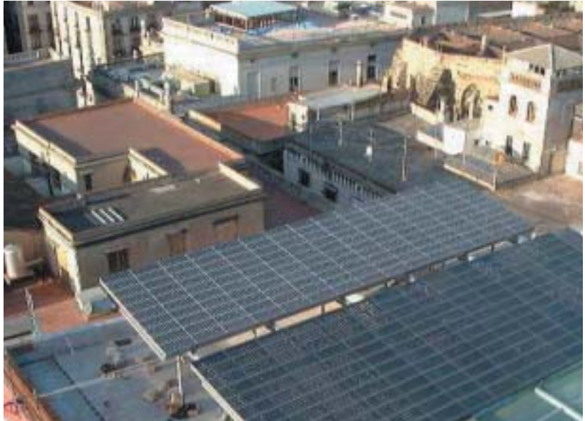
▲ Figure 7.4: Barcelona City Council roof installation. Source: Ajuntament de Barcelona.
