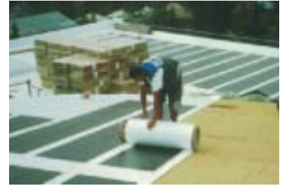
▲ Figure 6.12: Installation of solar membrane roof equals standard installation techniques. Source: Uni-Solar - Bekaert ECD Solar Systems LLC, Belgium; Picture: Alwitra GmbH, Germany.
