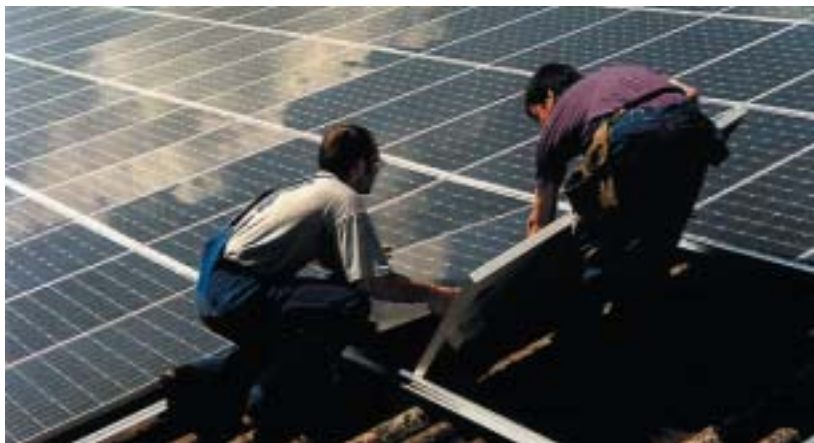
◀ Figure 2.1: To have a smooth procedure, photovoltaic integration should be considered from the very start of a project. Solar panels are mounted onto the roof in Hünenberg, Switzerland. Installed power is 32.56 kWp and produces solar electricity equivalent to the electricity consumption of 8 "average" Swiss families. Source: Urs Bühler, Cham, Switzerland.
