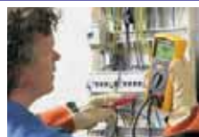
Insulation test at a distribution panel
